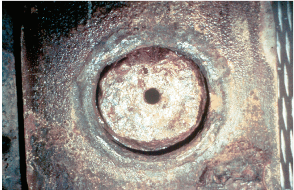
Figure 8.4.23 Corroded Pin and Hanger Assembly
