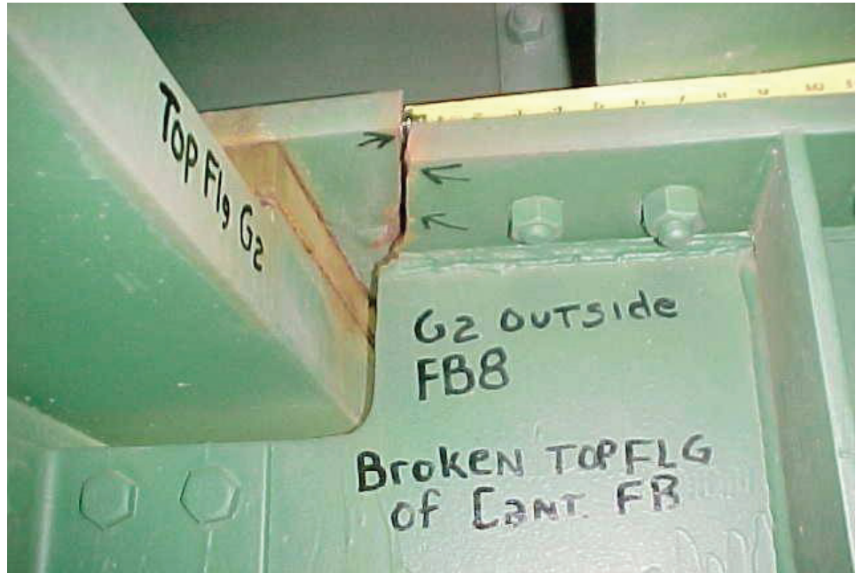
Figure 8.3.28 Cracked Cantilever Floorbeam
