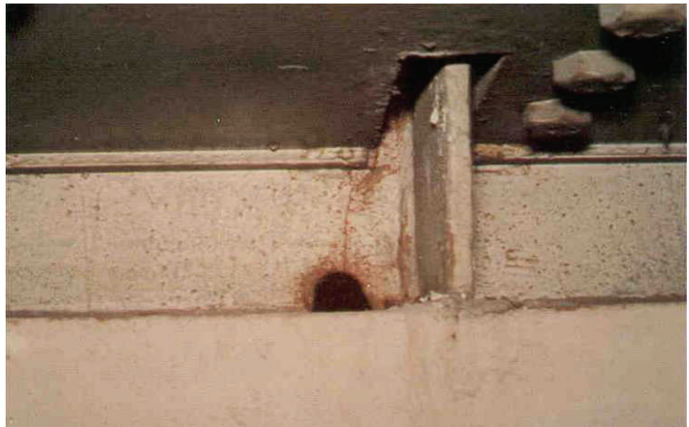
Figure 8.3.25 Crack Caused by Out-of-plane Distortion
