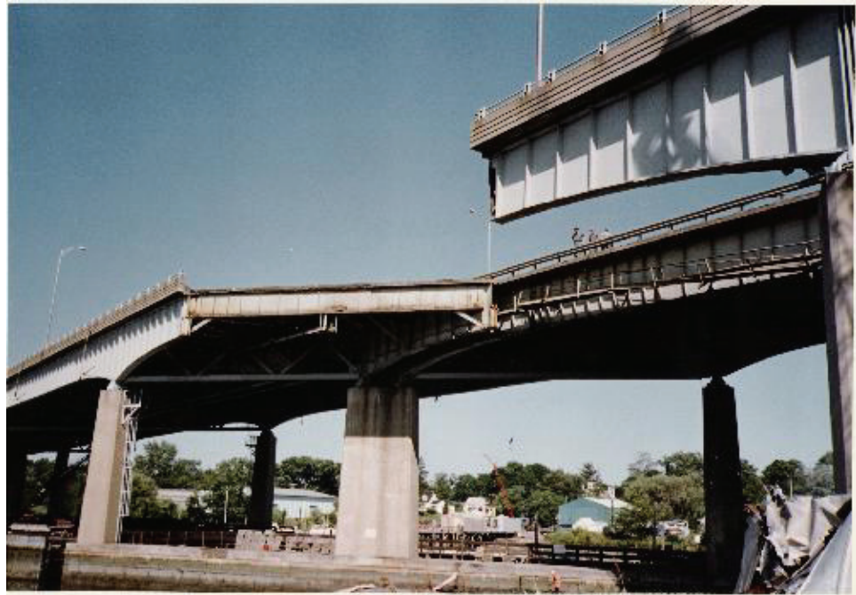
Figure 8.4.15 Mianus River Bridge Failure
