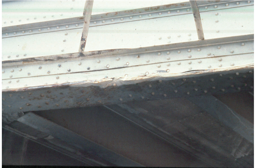
Figure 8.3.19 Collision Damage to a Through Girder Bridge
